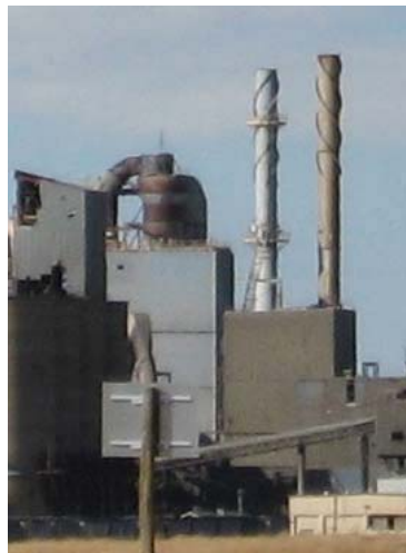
Figure 35. Helical strakes on stacks at the Mountain Cement Company in Laramie, WY
