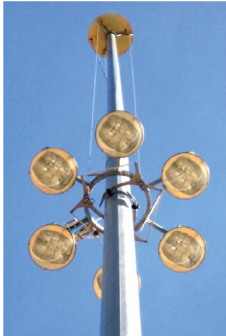
Figure 9. Ring assembly and luminaire on pole
