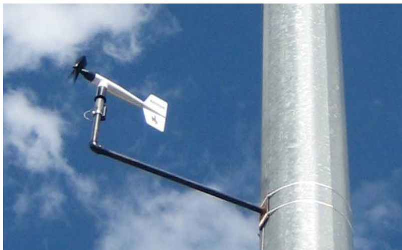
Figure 18. Anemometer mounted on high-mast pole
